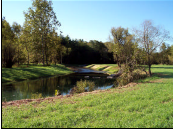
Photo 7, Post Construction: View looking downstream at constructed meander bend. Mature trees were left in place. The riffle-pool sequence was constructed to add diversity in the bottom profile of the stream.
