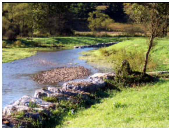
Photo 3, Post-construction: View looking downstream along the beginning of the re-constructed channel. Note the sloped banks with re-established grass, rock vane, and woody transplants to protect the streambank.
