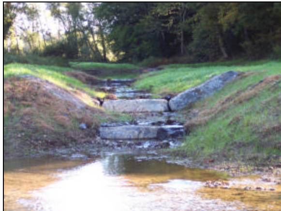
Photo 6, Post-construction: View shows a step-pool outlet channel carrying flow from a new wetland area back into the main channel. The step-pool channel was created using rock sills. The new wetland area was created from a portion of the original channel that had been straightened. The meander was reconstructed to bypass the old straightened channel.
