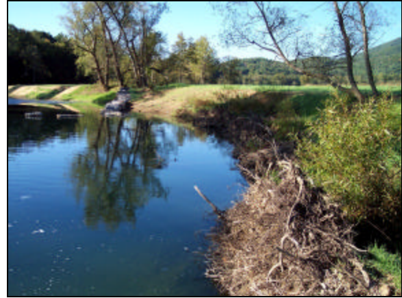
Photo 8, Post-construction (same meander bend as in Photo 7): Photo shows reconstructed portion of channel where the meander was restored. Natural design elements shown are the root wads, woody vegetation (willows), rock vane, and preserved mature trees. The rock vane will protect the bank and maintain pool depth for aquatic habitat diversity.
