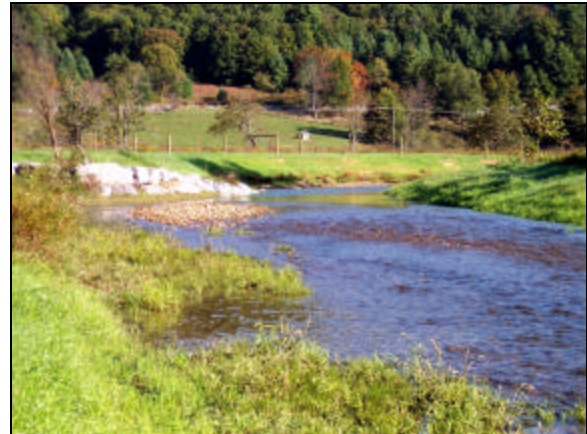
Photo 2, Post-construction (Same area as shown in Photo 1): View is looking upstream at the beginning of the reconstructed channel for Site 24. Natural stream design features include the sloped banks protected by seeding, woody transplants, fence to separate livestock from restored areas, reduced channel width, and a rock vane.
